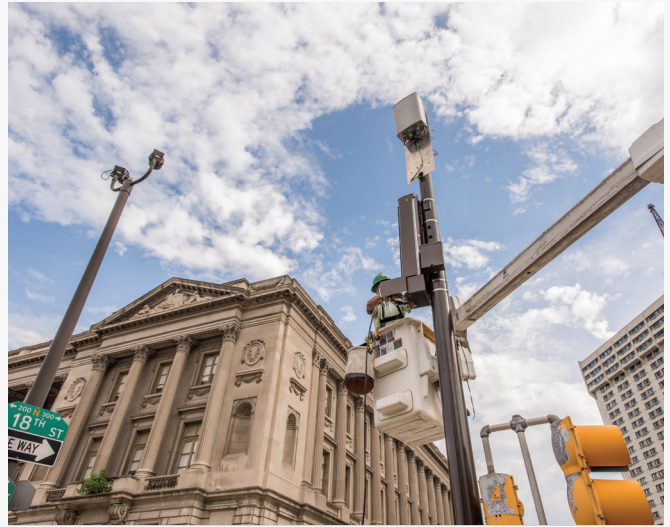
Small cells are installed on utility poles in Philadelphia.
