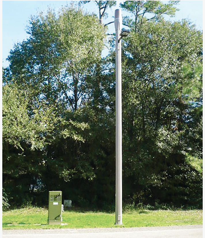
Small cell node installed on residential streetlight.
